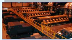
Diesel Power Plant
