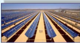
Solar Power Plant
